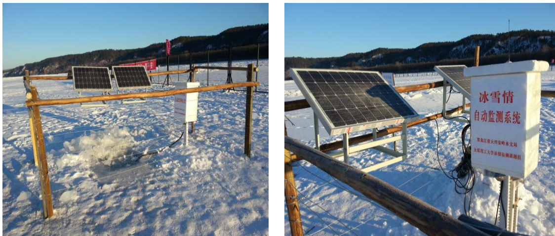
Figure6. The R-T Ice Automatic Measurement Sensor installed in Mohe , Heilongjiang river
